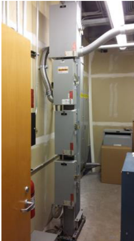
Figure VI-2. Typical Bus Duct Riser in Electrical Rooms
