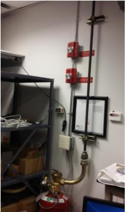
Figure VI-3. FM-200 Fire Suppression System
