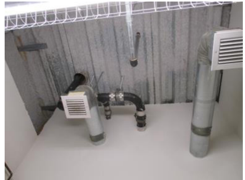
Figure III-1. Support space ceiling exhaust grilles.
