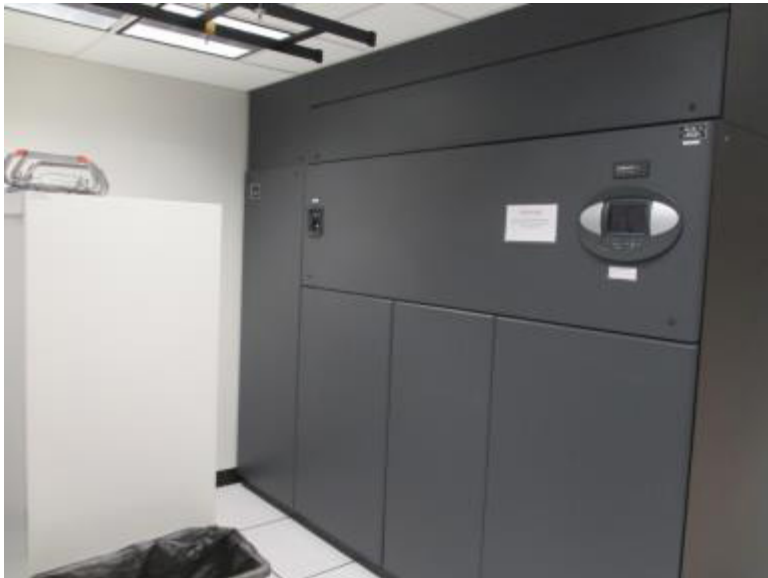
Figure III-2. Dedicated CRAC unit.
