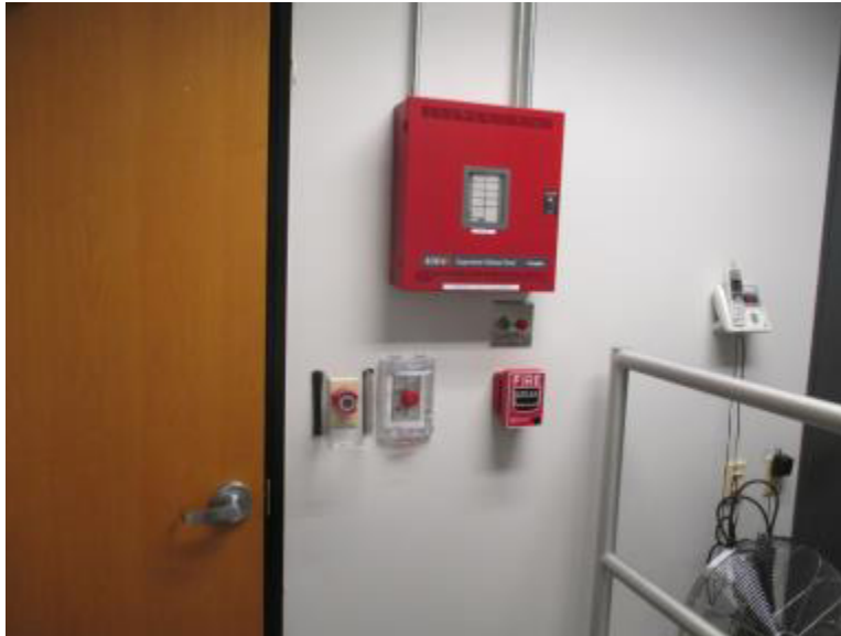
Figure V-1. FM200 system components.
