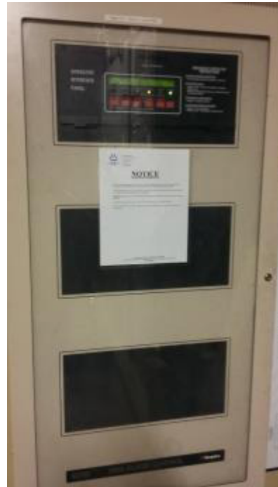
Figure VI-7. Fire Alarm Control Panelboard
