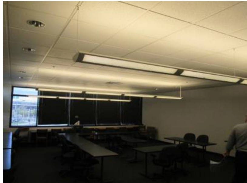
Figure VI-6. Typical Conference Room Lighting
