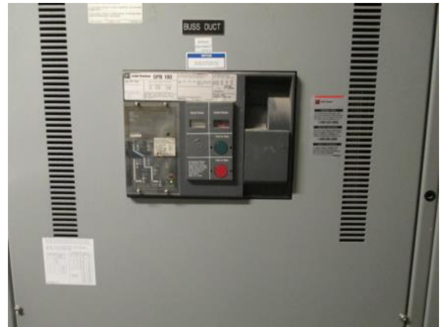
Figure VI-1. 2,000 Amp Bus Duct Overcurrent in MDC
